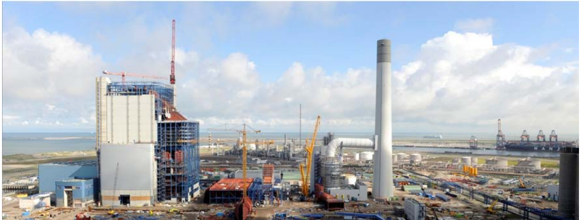
Location of the capture unit: Maasvlakte Power Plant 3 (photo: E.ON)
