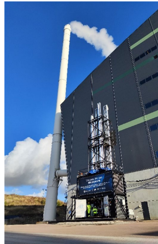
CapsolGo® unit 1 at Filbörnaverket, Helsingborg, Sweden.
