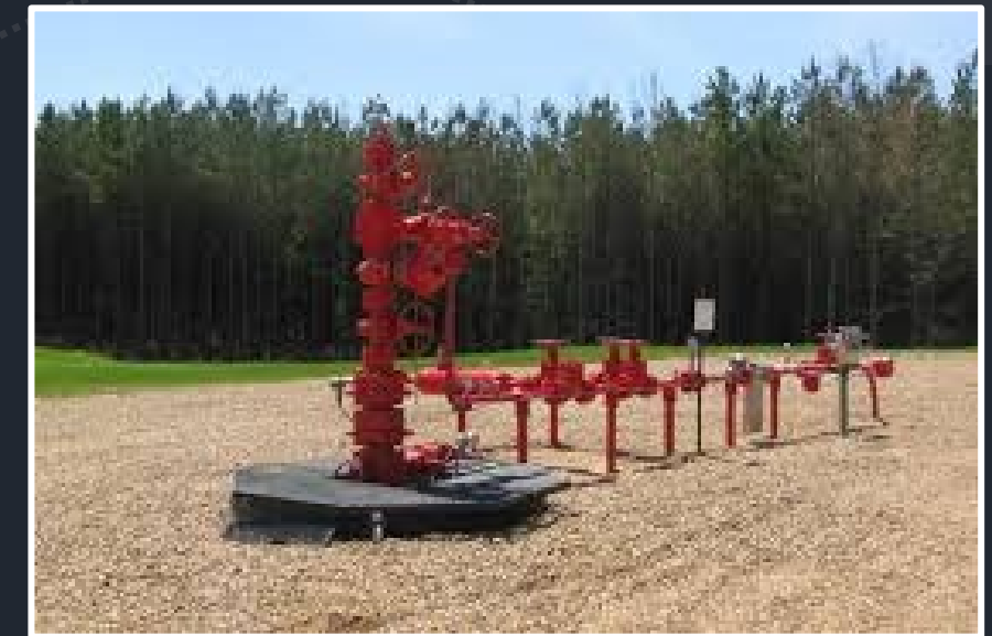
CO 2 Injection Well
