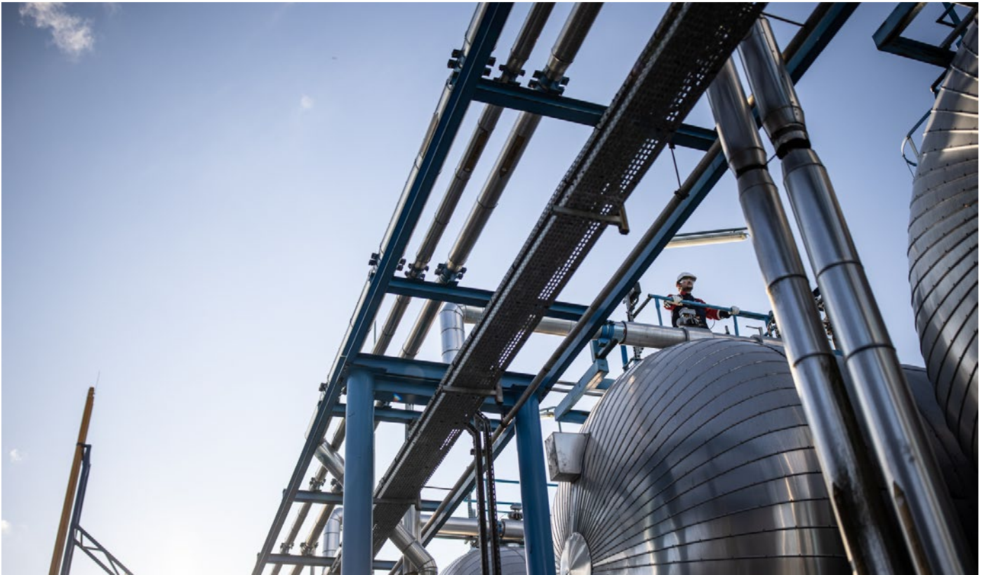
Port-Jerome. Credit: Air Liquide
