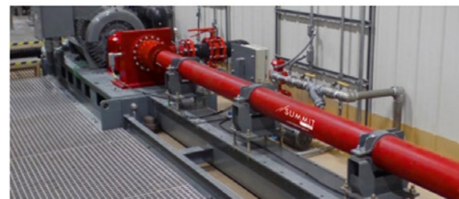
Produced Salt Water Disposal (400 hp / 12,000 bpd / 1,250 psi)
