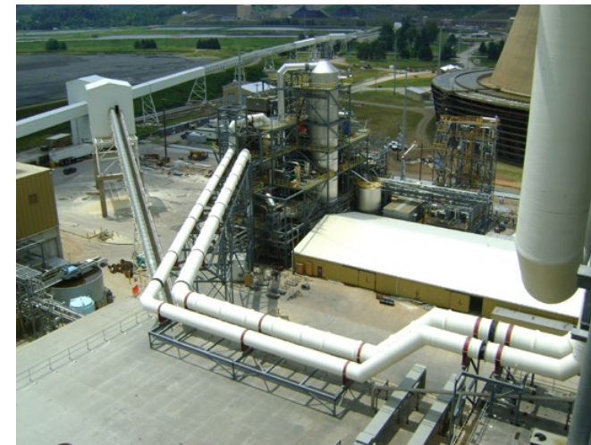
American Electric Power (AEP) Mountaineer Station
