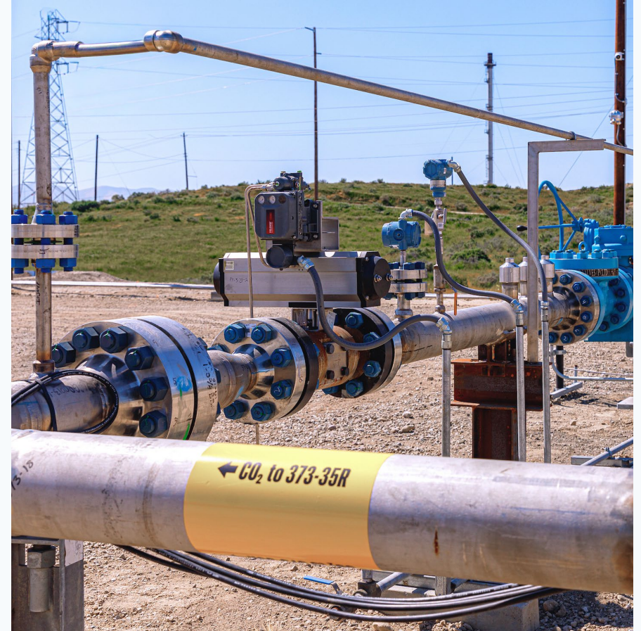
Carbon TerraVault I (CTV-1) storage well. Image courtesy of California Resources Corporation.
